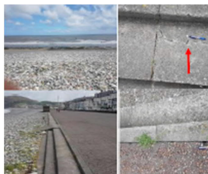
Photo 2: Moderately abrasion to concrete surface revetment
