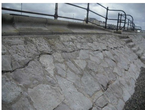
Photo 1: Cracking in Wall to Paddling Pool
