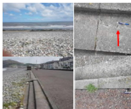
Photo 2: Moderately abrasion to concrete surface revetment
