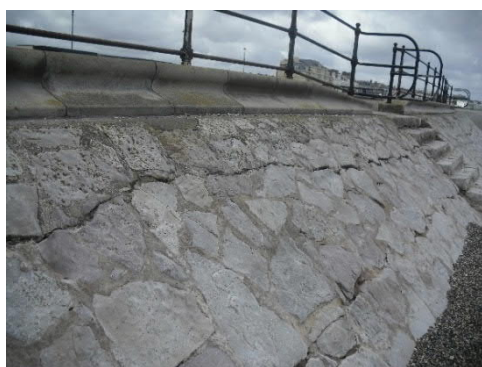
Photo 1: Cracking in Wall to Paddling Pool
